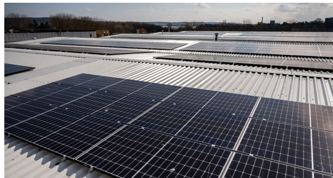
Solar panels installed on the roof of the Holophone production facility in Milton Keynes, United Kingdom will allow the facility to provide up to 80% of its annual electrical power consumption and return an estimated energy surplus of 45,000 kWh per year to the grid.
